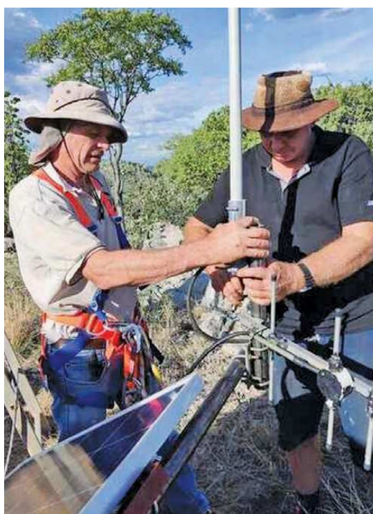
Olaf Bucking, V51OB, and Robert Schenk, V51RS, begin work on the antennas for the Outjo repeater. [Namibian Amateur Radio League photo]
