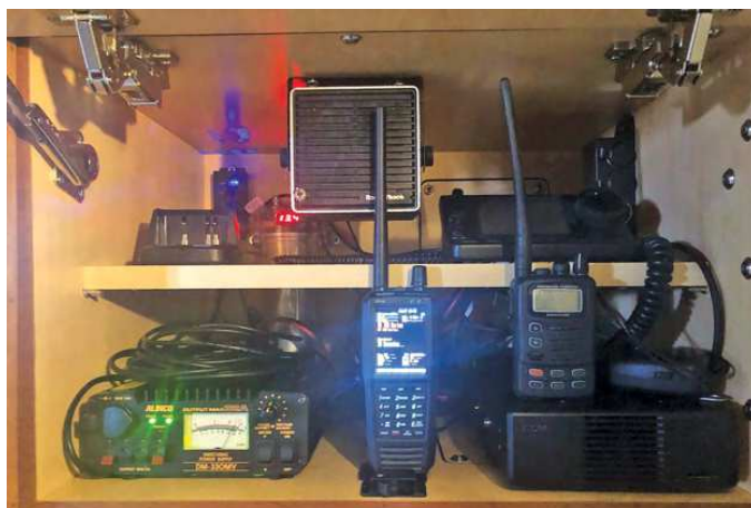
The radio cabinet is home to handhelds, accessories, and other necessities.
